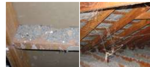
5. Building cavities A small number of homes may still contain loose fill asbestos insulation in the roof cavity, wall cavities or sub-floor space
