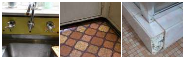
2. Wet areas - bathroom, laundry and kitchen wall and ceiling panels, vinyl floor tiles, backing for wall tiles and splashbacks, hot water pipe insulation
