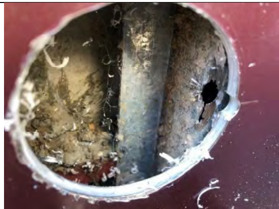
Photo 11: Sample 122535 – behind panel
