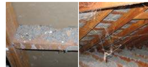
5. Building cavities A small number of homes may still contain loose fill asbestos insulation in the roof cavity, wall cavities or sub-floor space
