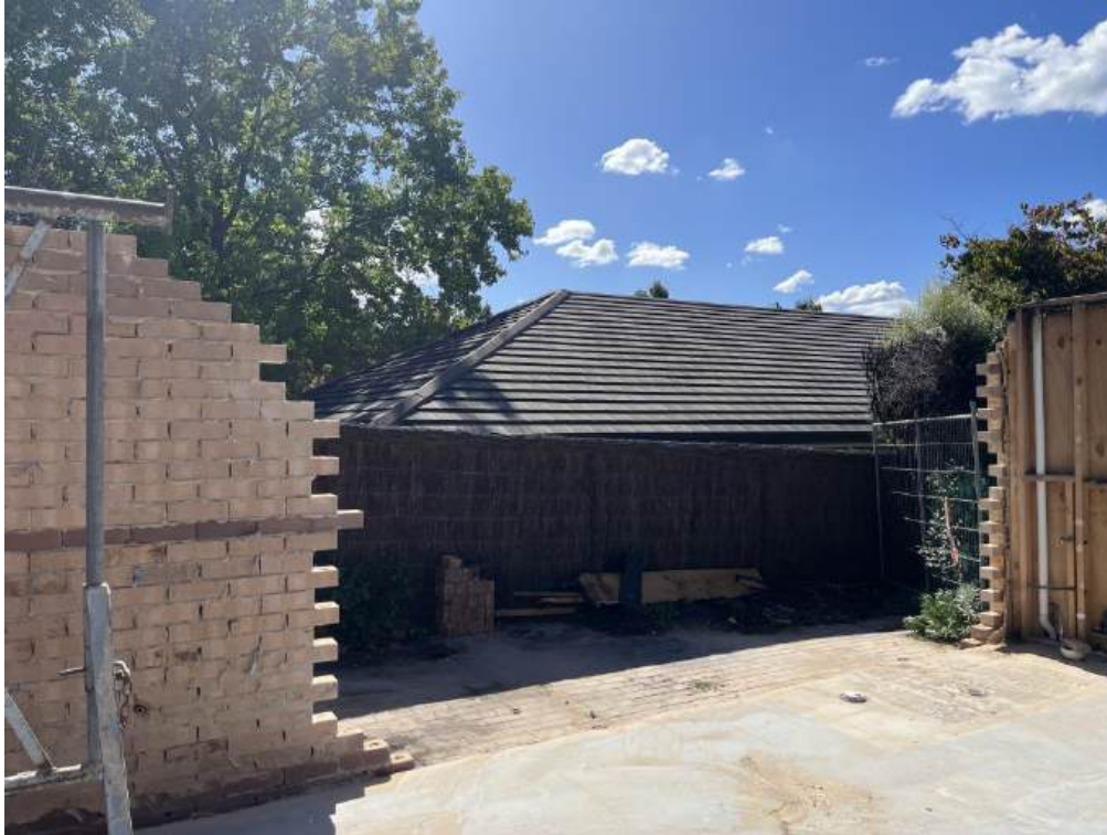
Image 2. View of the Existing Brickwork to Remain and New Brickwork to Integrate and Tooth Into
