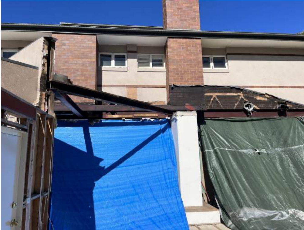
Image 1. View of the Exposed Beams and Soot/Smoke Affected Brickwork
