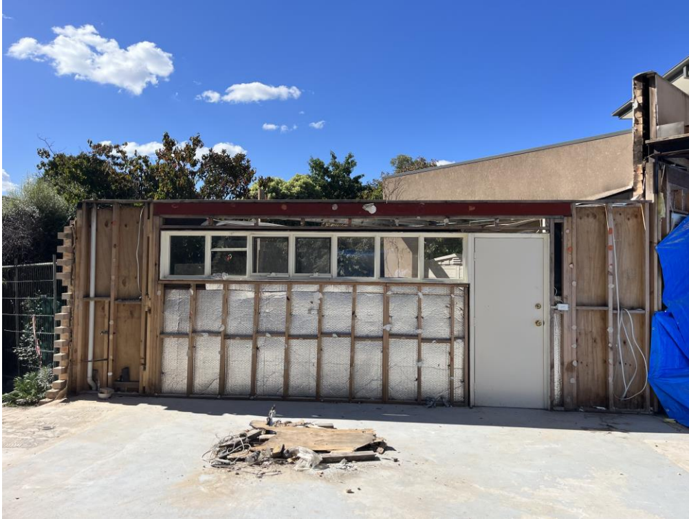
Image 3. View of the Brick Veneer Timber Stud Work to Removed and Replaced, Veneer to Remain in Place
