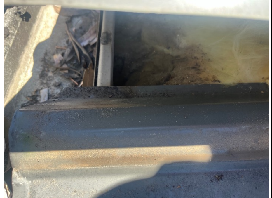
Photo 1.13 Tag to underlap of roof sheet
