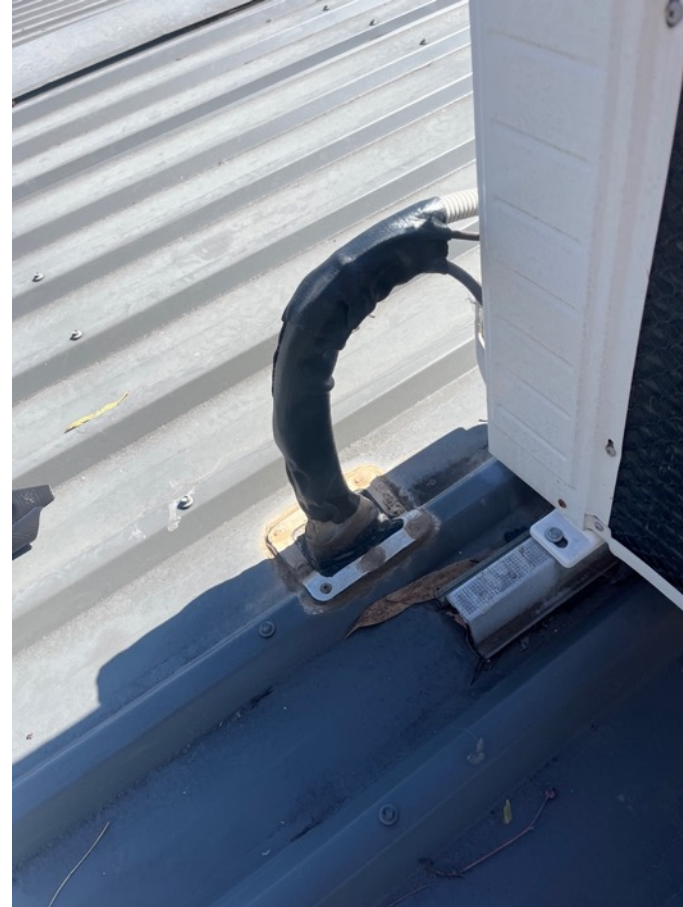
Photo 1.11 Polymer sheath to air conditioning grouped services
