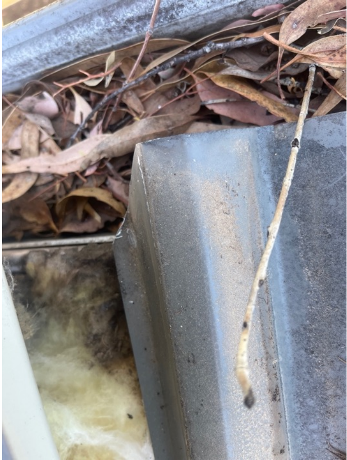
Photo 1.12 Tag to underlap of roof sheet
