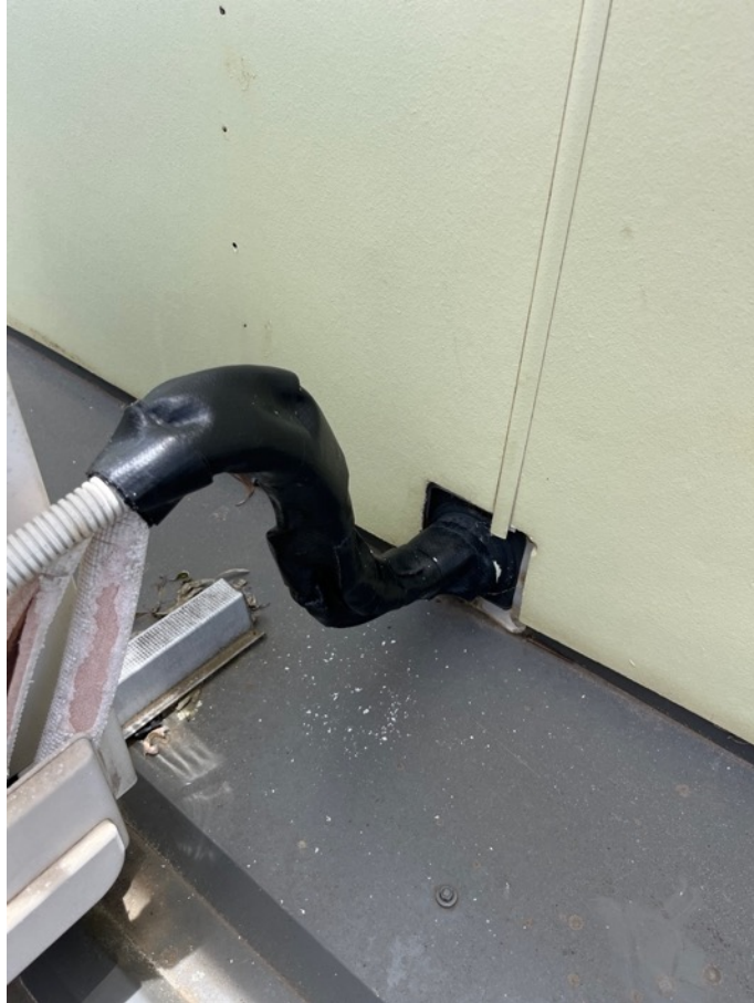
Photo 1.10 Polymer sheath to air conditioning grouped services
