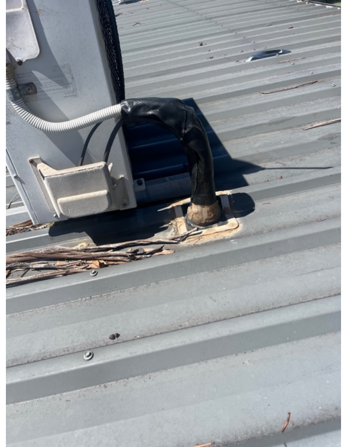
Photo 1.9 Polymer sheath to air conditioning grouped services
